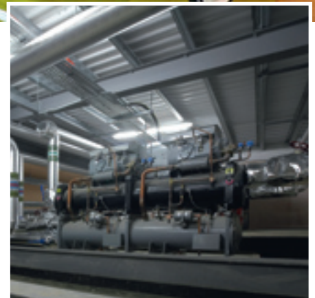
VRF heat exchange system
